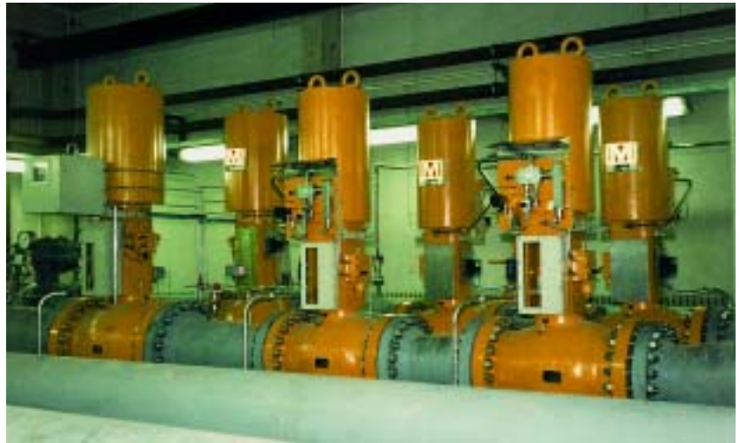
pressure control valves 20" ANSI 600 lbs and safety slam shut valves 16" ANSI 600 lbs, M & R station Germany
