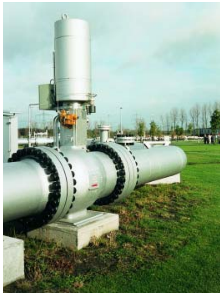
HIPPS valve 28" ANSI 600 lbs in natural gas booster station, Germany
